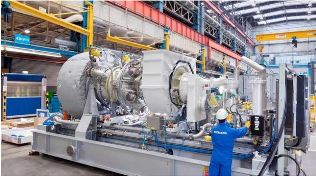
Figure 2.6: A section of an Industrial gas turbine, within the Wang Noi compressor station in Thailand (SGT-400 industrial gas turbines Courtesy Siemens Power Generation).
