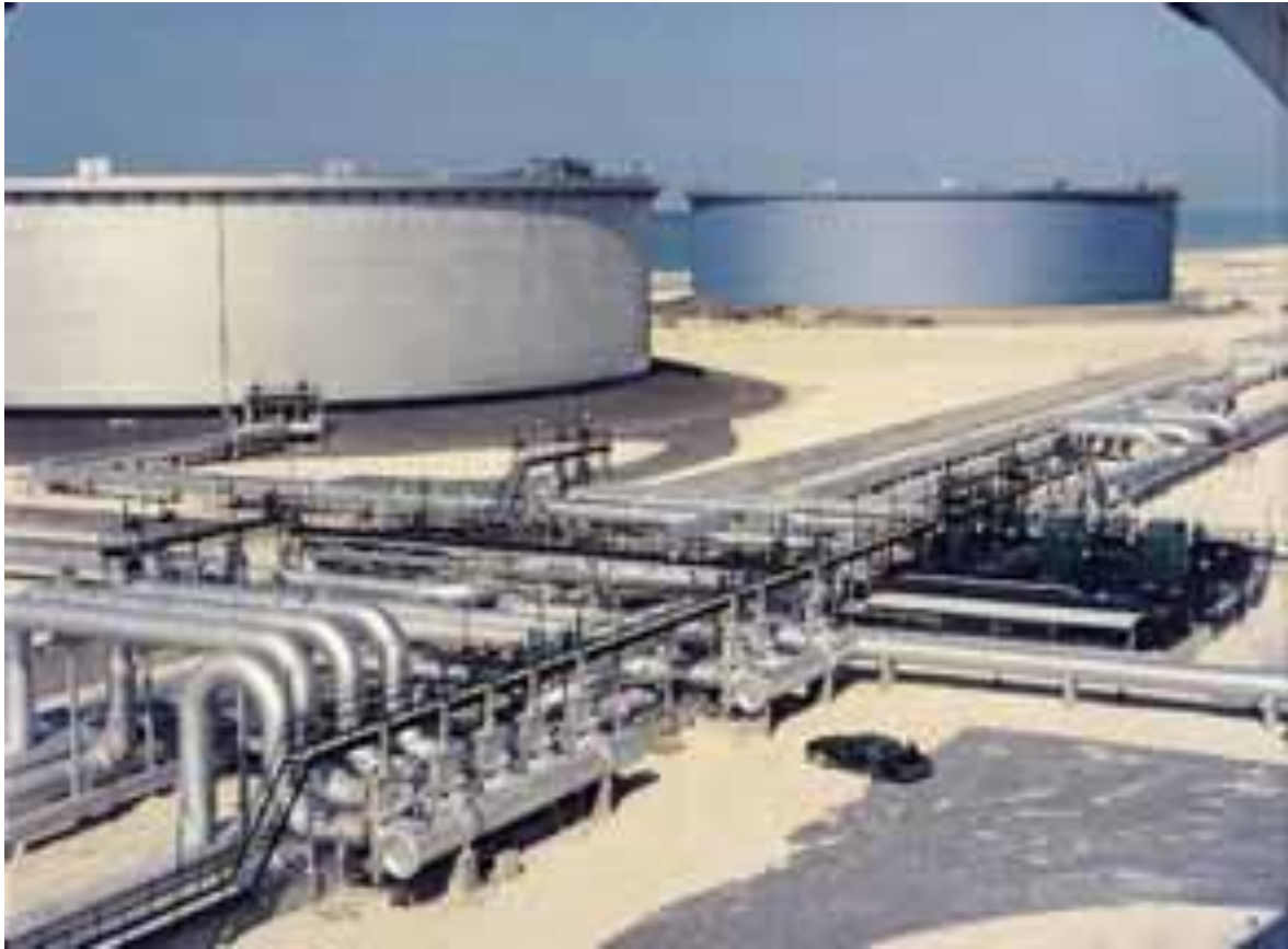
Plate 2.7: Crude Oil Storage Tank (Devold, 2013).
