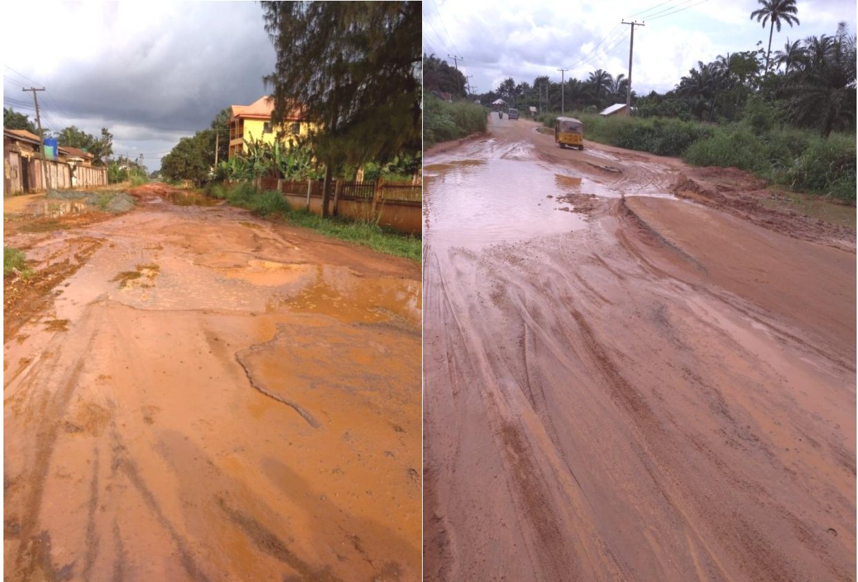
Plate 1.1: Severe Potholes and Ponding Water on Potholes at (A) Amanachi and (B) Isseke (Orsu-Ihiala road).
