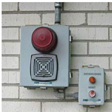
Figure 2.6: Audible and strobe overfill alarm
