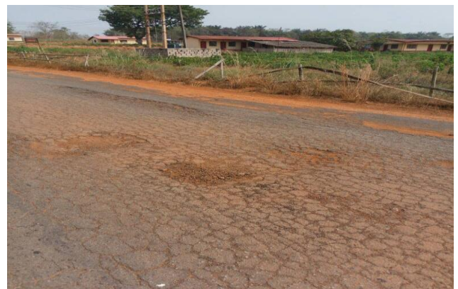
Figure 1.4: Failed portion of the road at Ufuma
