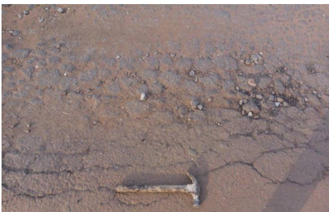
Figure 1.3: Failed Portion of the road at Enugwu- Agidi
