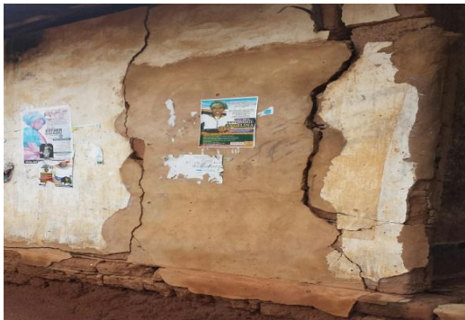
Figure 1.1: Abandoned building due to cracks at Ugwuoba
