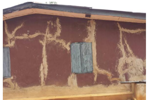
Figure 1.2: Patched cracks on the wall due to expansive soil at Ugwuoba
