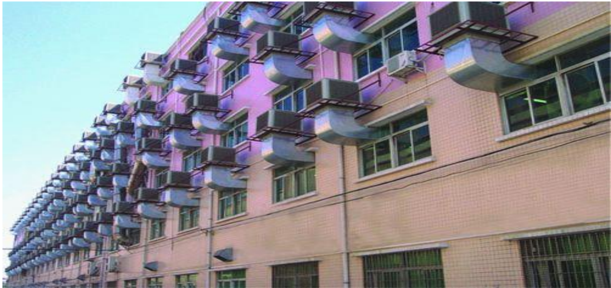
Figure 2.13 Multiple evaporative coolers installed on a factory building (Muazu, 2008).
