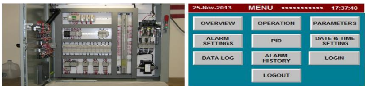
Plate 2.33: PLC Panel and HMI (Rakshe, 2017)
