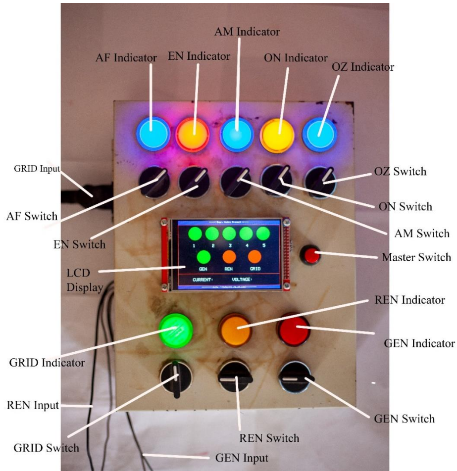
Fig. 3.18: The hardware assembly of the Intelligent Master Controller
