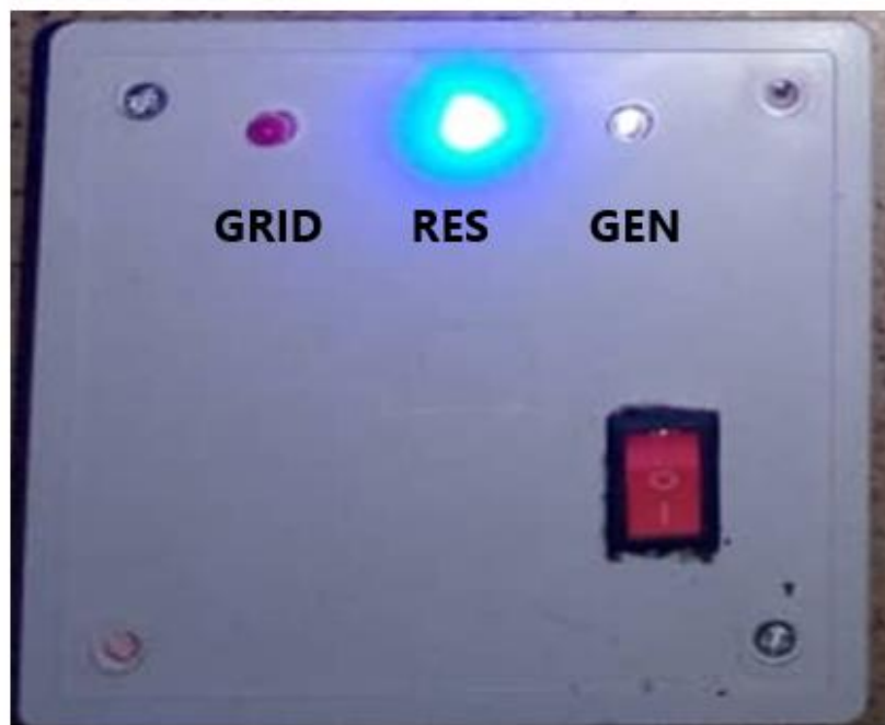
Fig. 3.20: Multiple Automatic Generator Starting assembly
