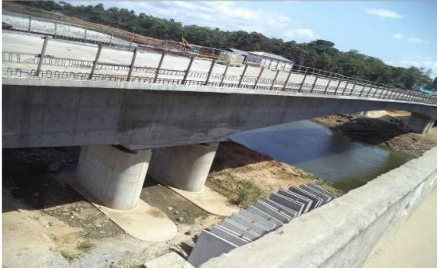
Plate 3.2: Stream Cut-across by an Overhead Bridge around Okujagu Community at the Trans-Amadi Industrial Layout in Port Harcourt
