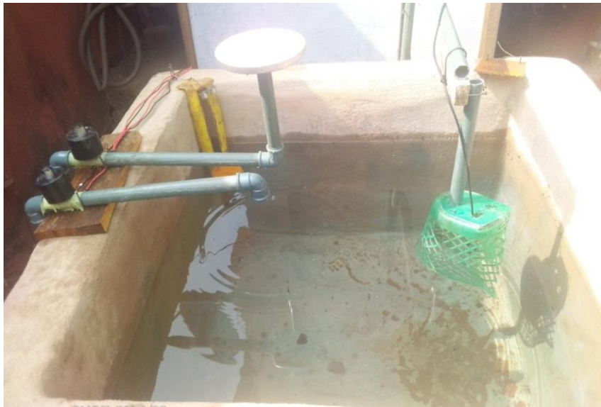
Plate 3.7: Snapshot of installed temperature and water level sensors and valves
