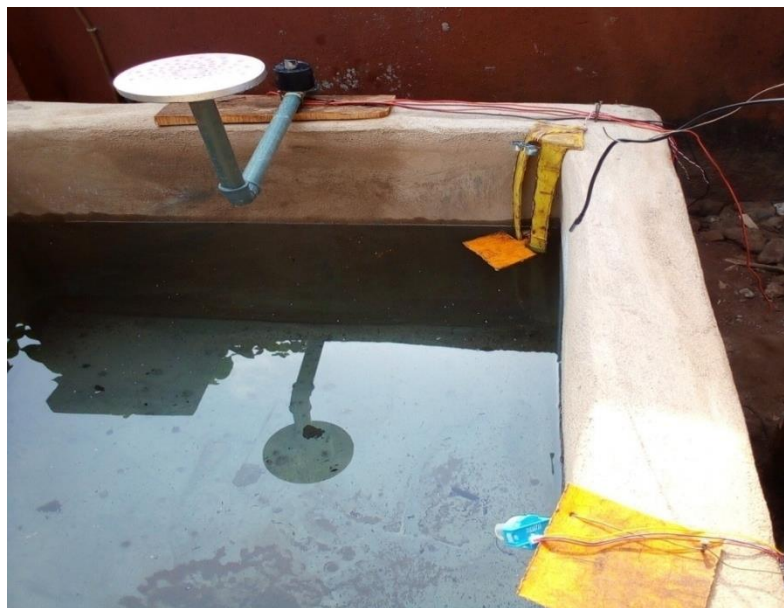
Plate 3.17: Snapshot of installed turbidity, temperature and water level sensors and valve
