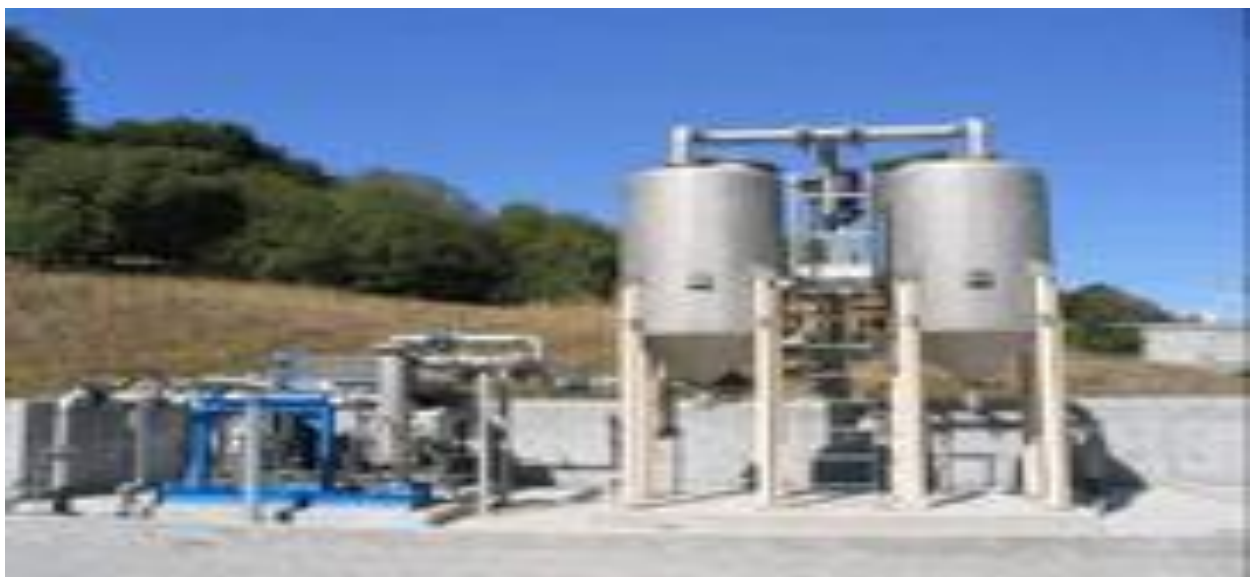
Fig 2.6: CNG Production Units
