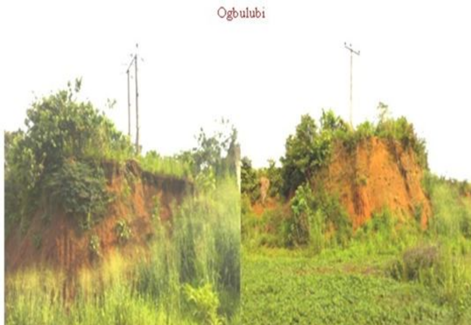
Plate 7: High tension pole hanging at the crest of an abandoned borrow pit, may collapse by the next sliding
