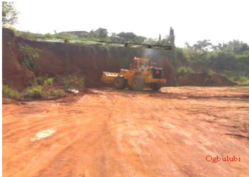
Plate 6: Family home; a duplex, fence threatened to collapse by next sliding as excavation still goes on
