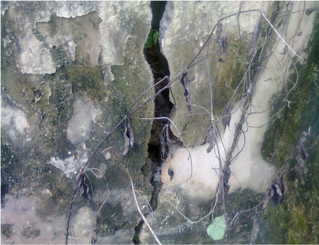
Plate 4c: Cracked buildings within Awgu area (study location)
