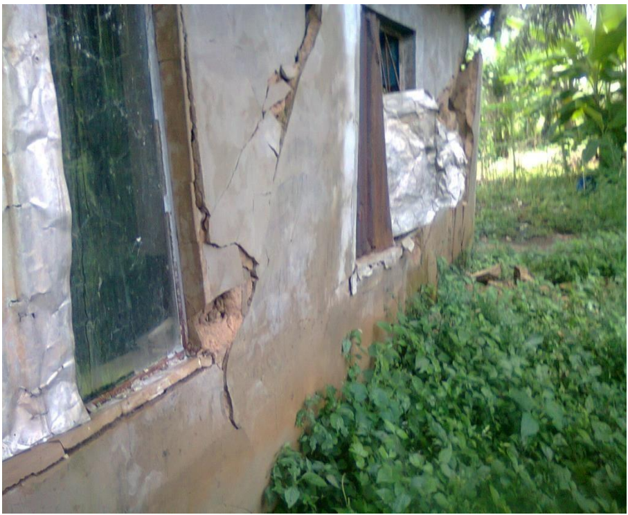
Plate 4b: Cracked buildings within Awgu area (study location)
