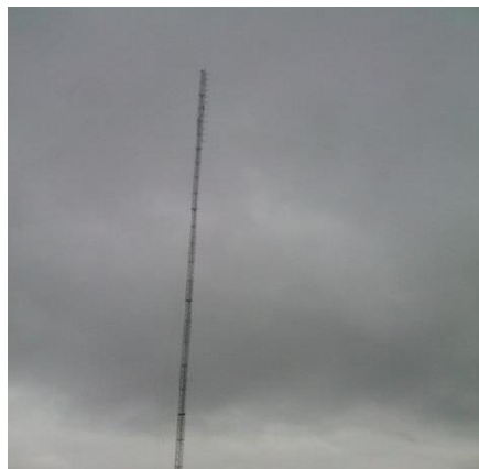
Fig 2: Guyed type antenna structure (courtesy:Radio Nigeria-Heartland FM, Owerri)
