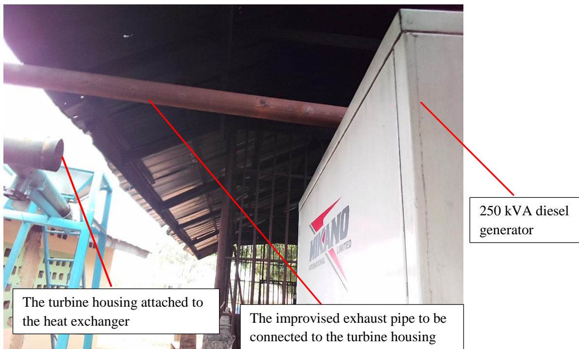
Plate 3.4: The point of connection of the turbine housing to the 250kVA generator set
