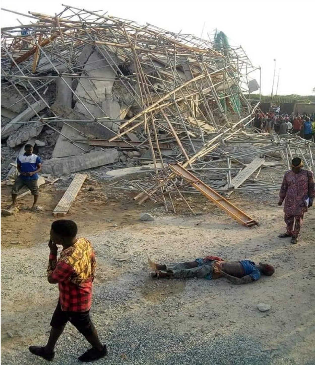
Plate 9: 8 – Storey Building under construction that collapsed at Yardua Drive Owerri (April 30, 2020). Source; www.google.com.ng
