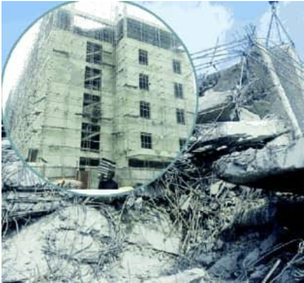
Plate 6: 7 – Storey Building collapse in Port Harcourt. Source: www.google.com.ng
