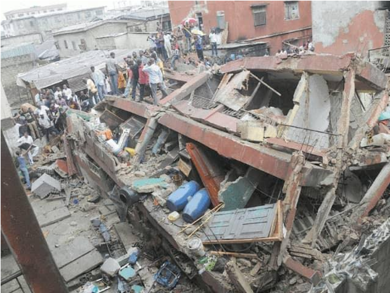
Plate 5: Collapse of a 2 – Two Storey Building Bode Area of Ibadan Source: www.google.com.ng
