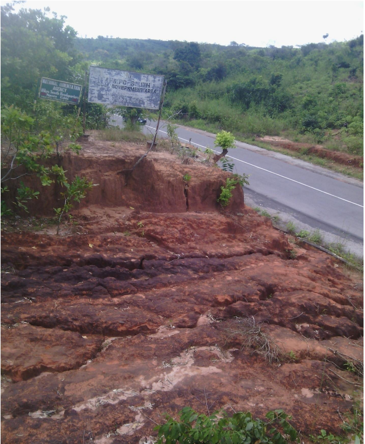
Plate B3- Access Road to Nguzu Edda Erosion Site 2
