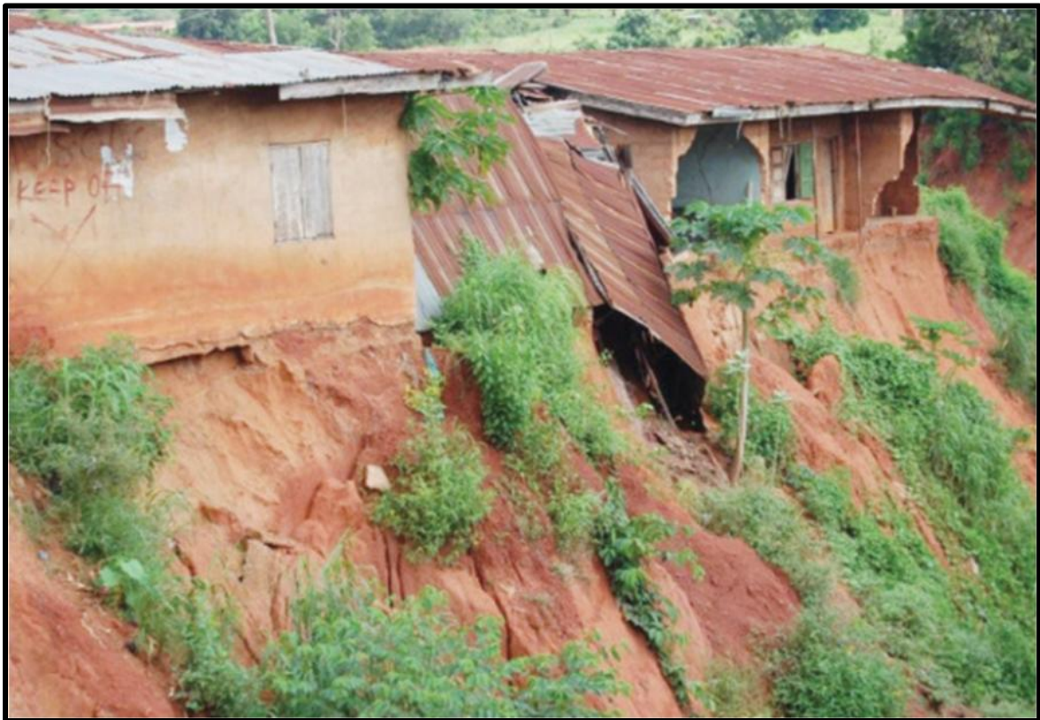
Plate 1. Destroyed building at Umueshi in Ideato North L.G.A of Imo State.
