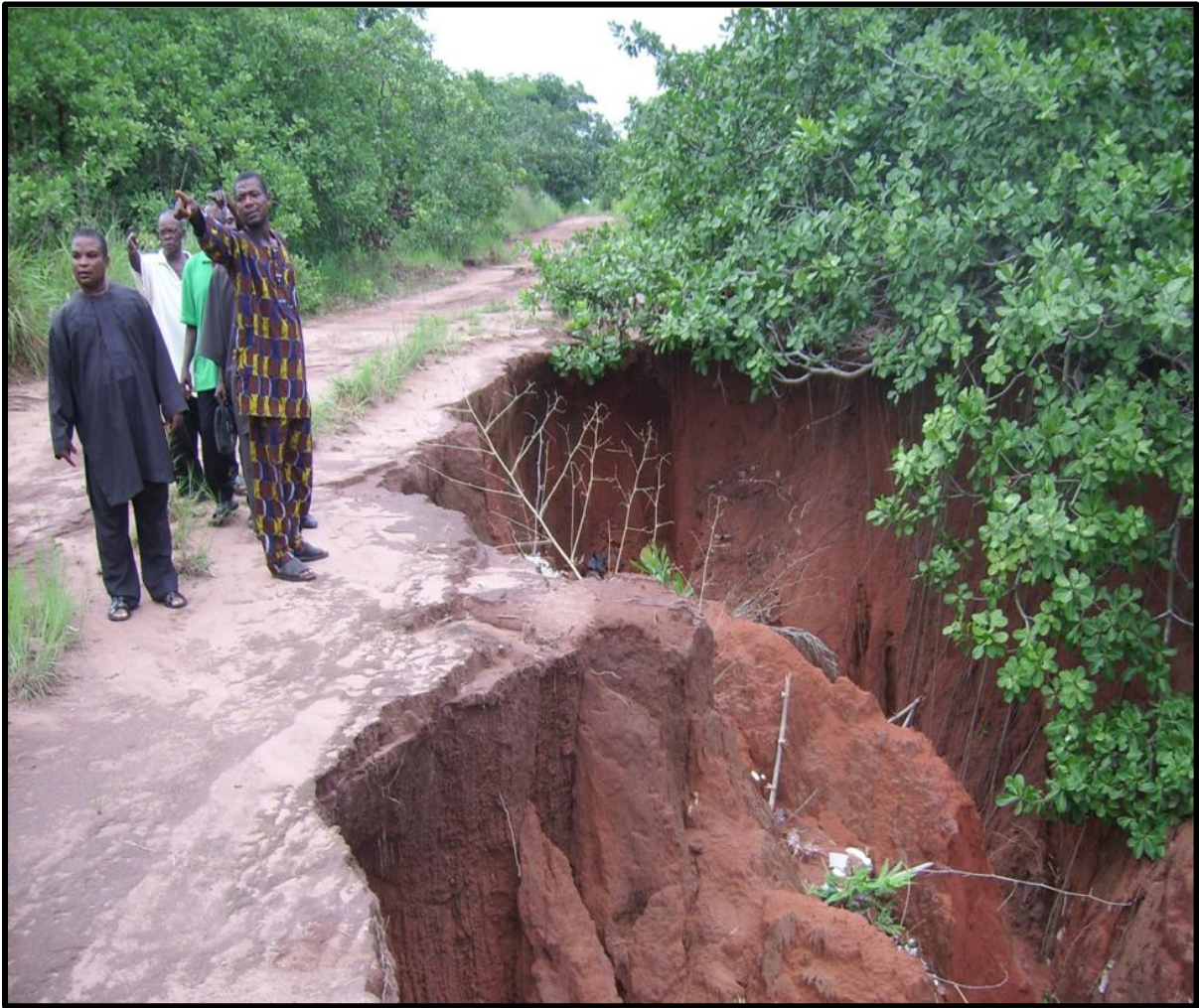
Plate 3. Destroyed road at Ogberuru, in Orlu.
