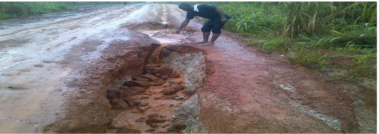
Plate 4: Water eroding the soil in Umuduru Okigwe L.G.A
